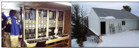
Figure 7.37 Camera control units and camera remote control panels in a secondary compound up on a mountain. From here, camera feeds are multiplexed onto fiber and sent down to the production trucks in the main compound. (Source: Chadwick Wachs)
